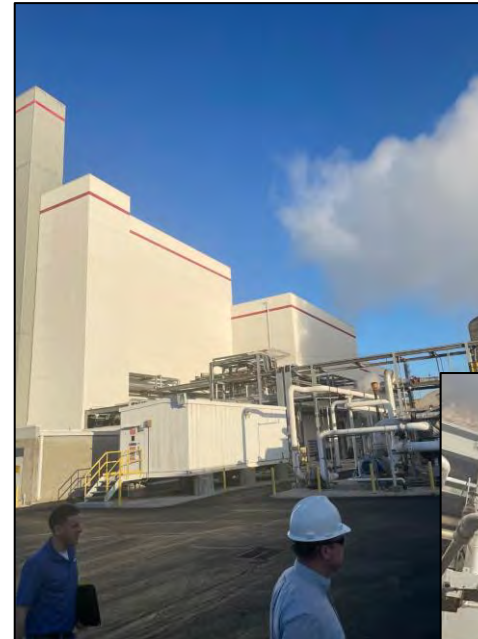
Orlando Cogeneration Facility
