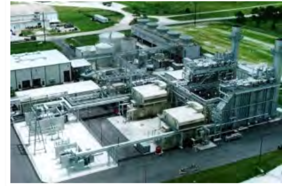
Orange Cogen Facility
