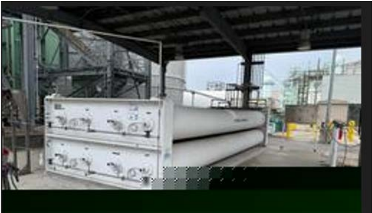
Cane Island Unit 4 H2 Storage System
