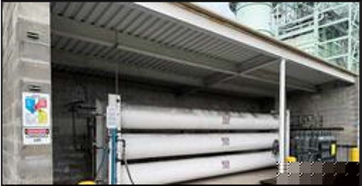
Cane Island Unit 3 H2 Storage System
