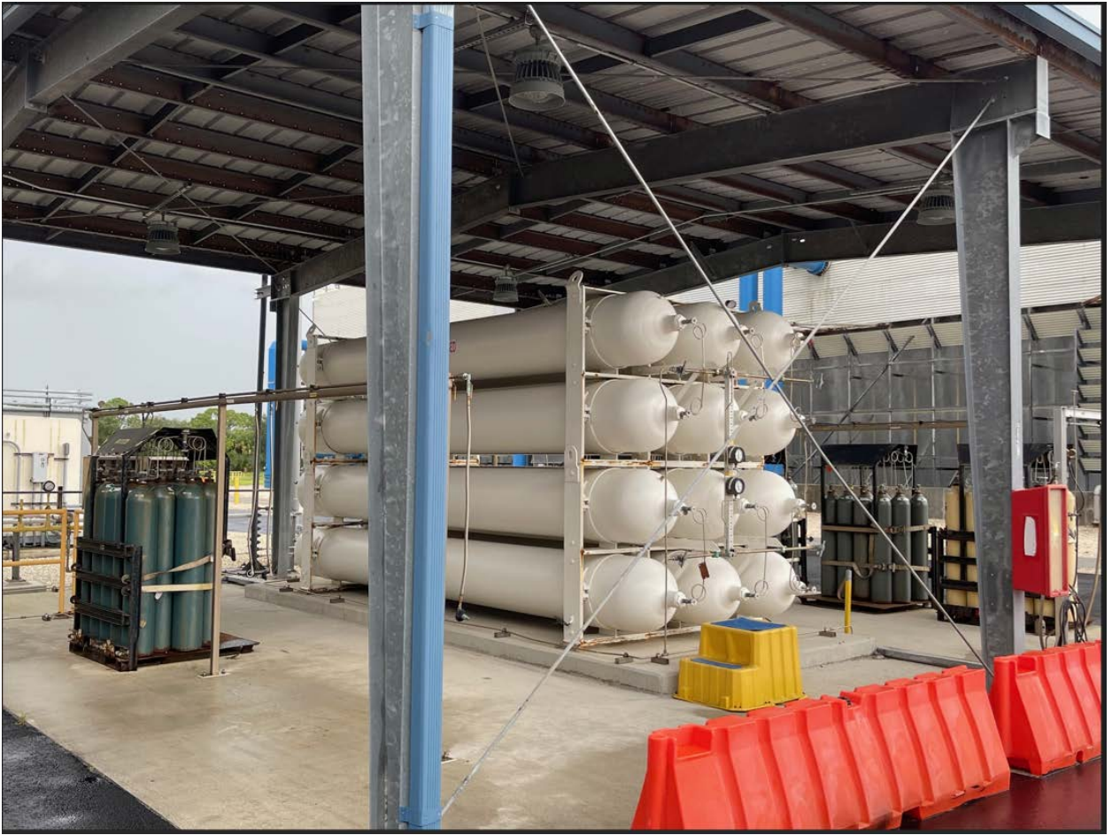
Treasure Coast unit 1 H2 Storage System
