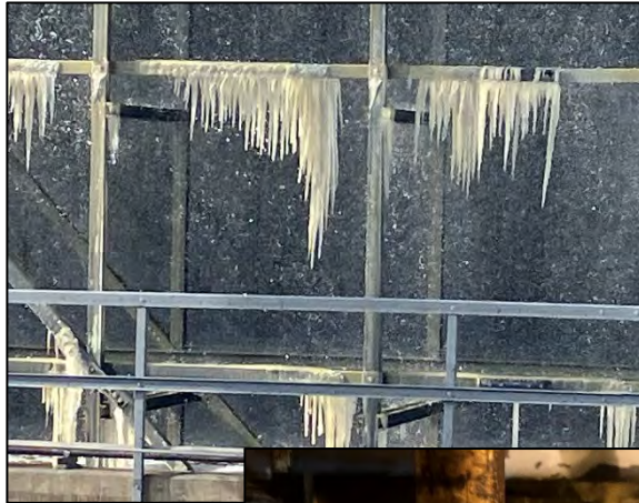
Ice on Cane Island equipment created challenges for repairs
