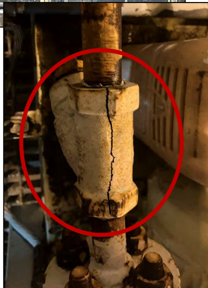
Iron piping froze and cracked
