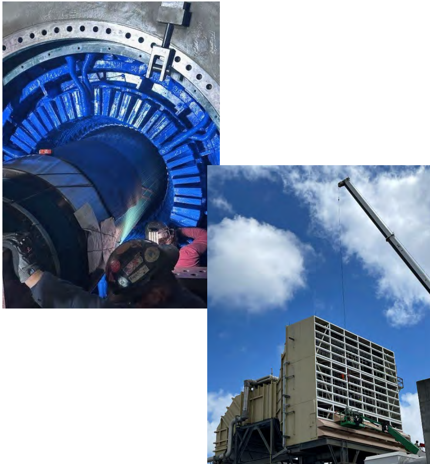
CT Generator Repair Completion Delayed Inlet Repair
