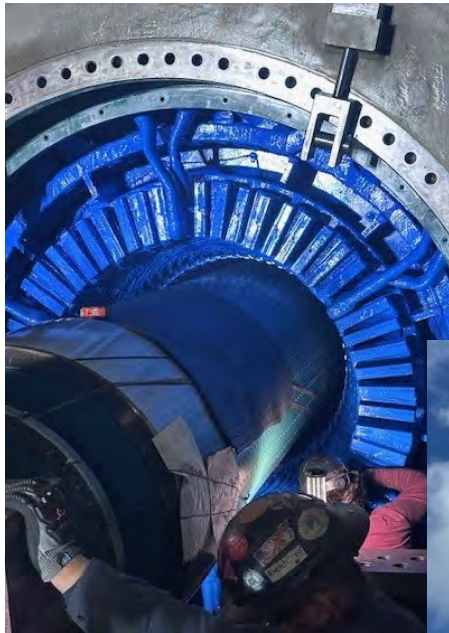
CT Generator Repair Completion Delayed Inlet Repair
