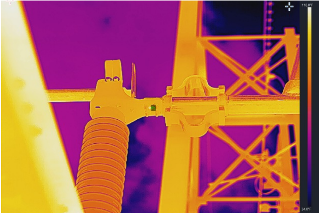
T1 - MAIN AIR SWITCH
