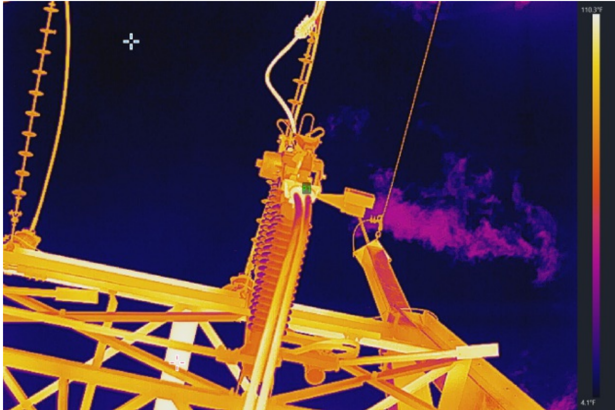
SWITCHYARD MAIN SWITCH
