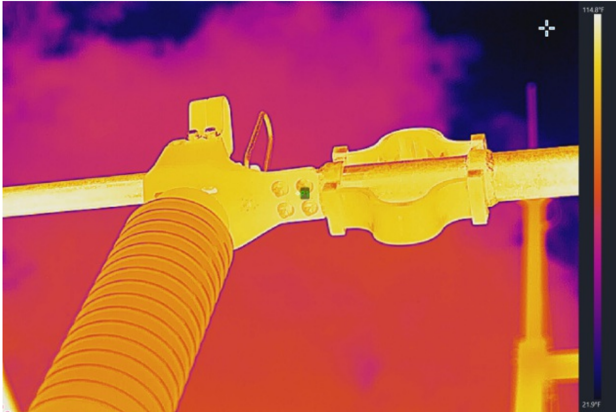
T1 - MAIN AIR SWITCH
