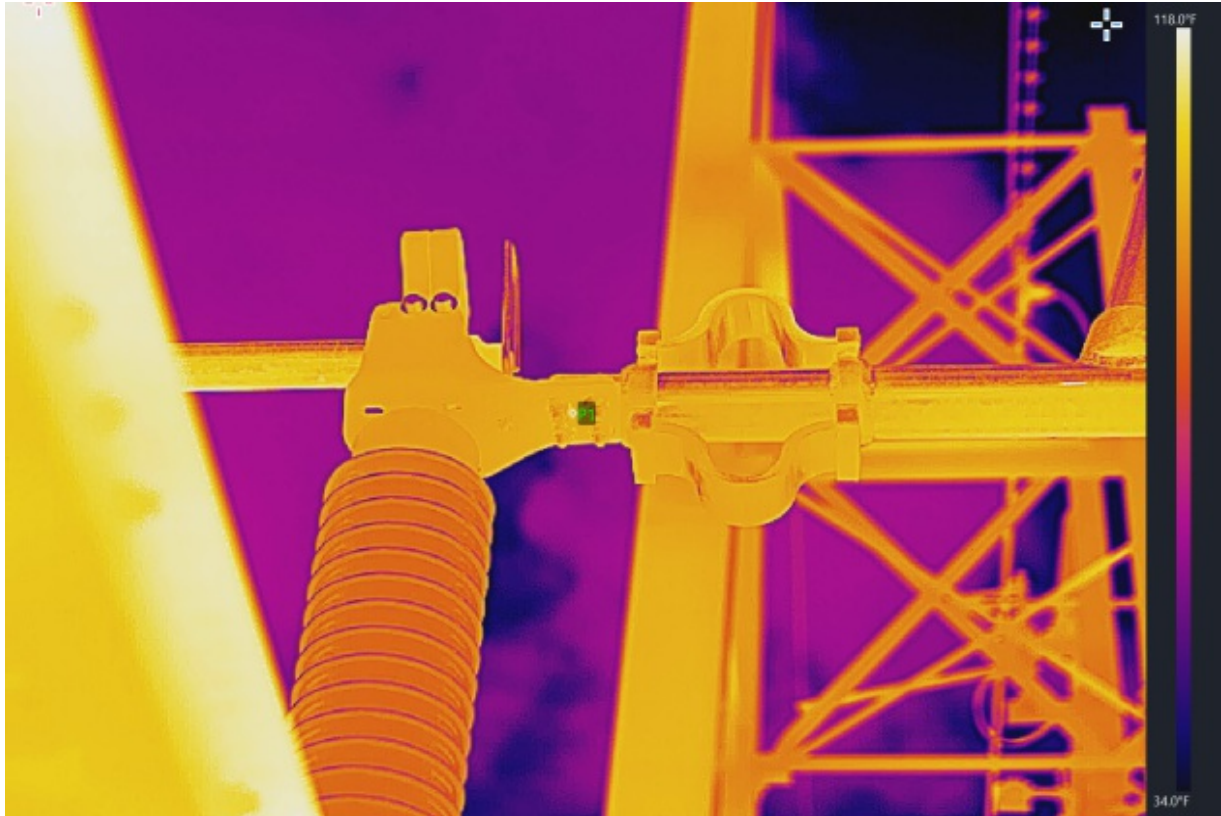
T1 - MAIN AIR SWITCH
