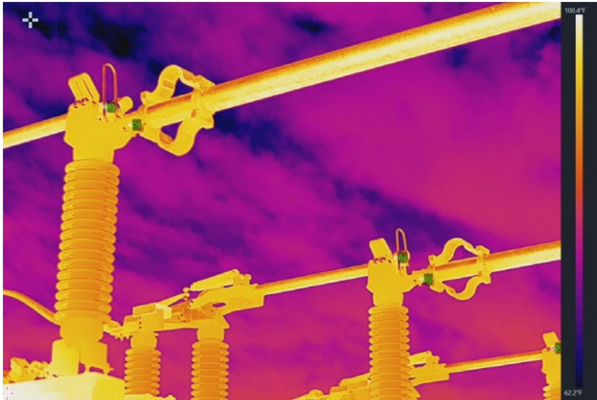
T1 - MAIN AIR SWITCH
