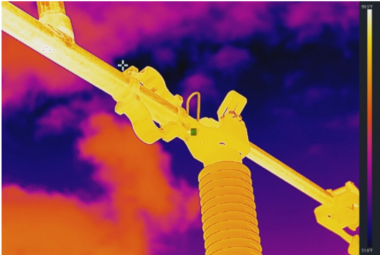
T1 - MAIN AIR SWITCH
