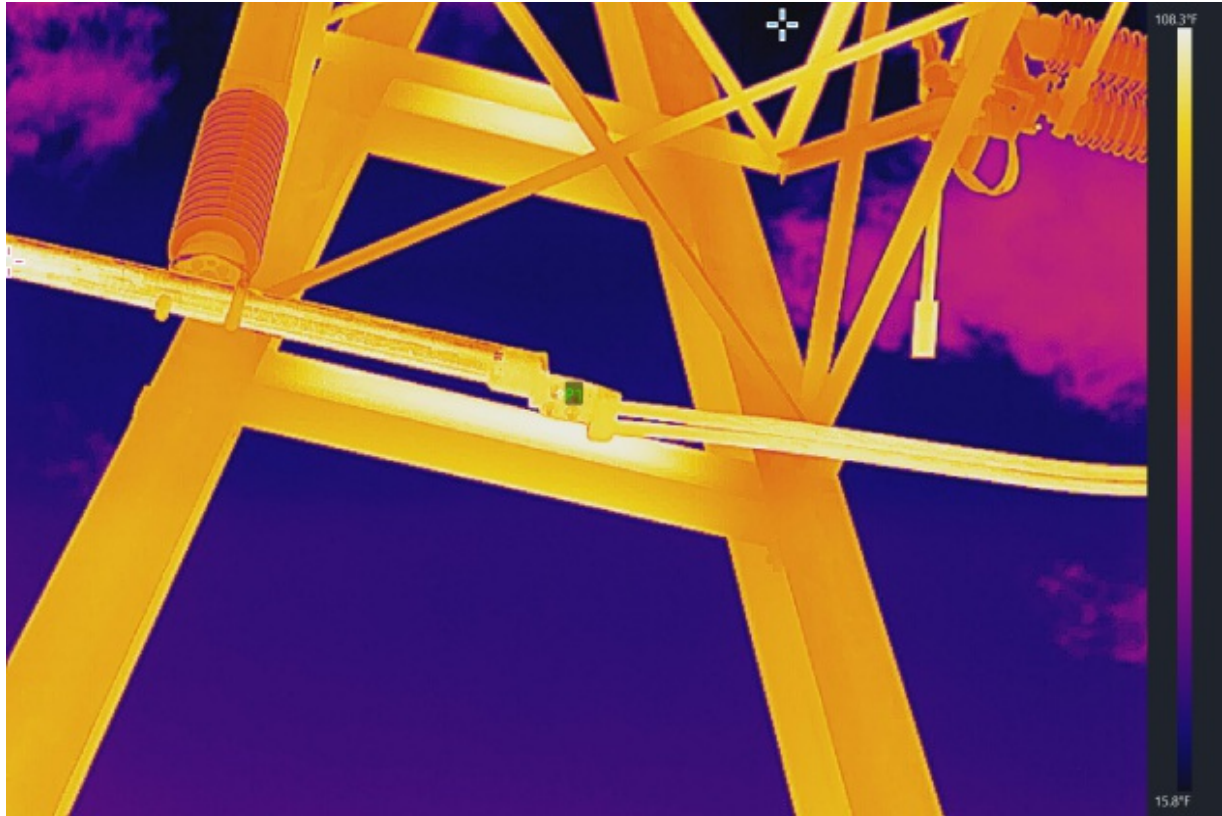
SWITCHYARD MAIN SWITCH
