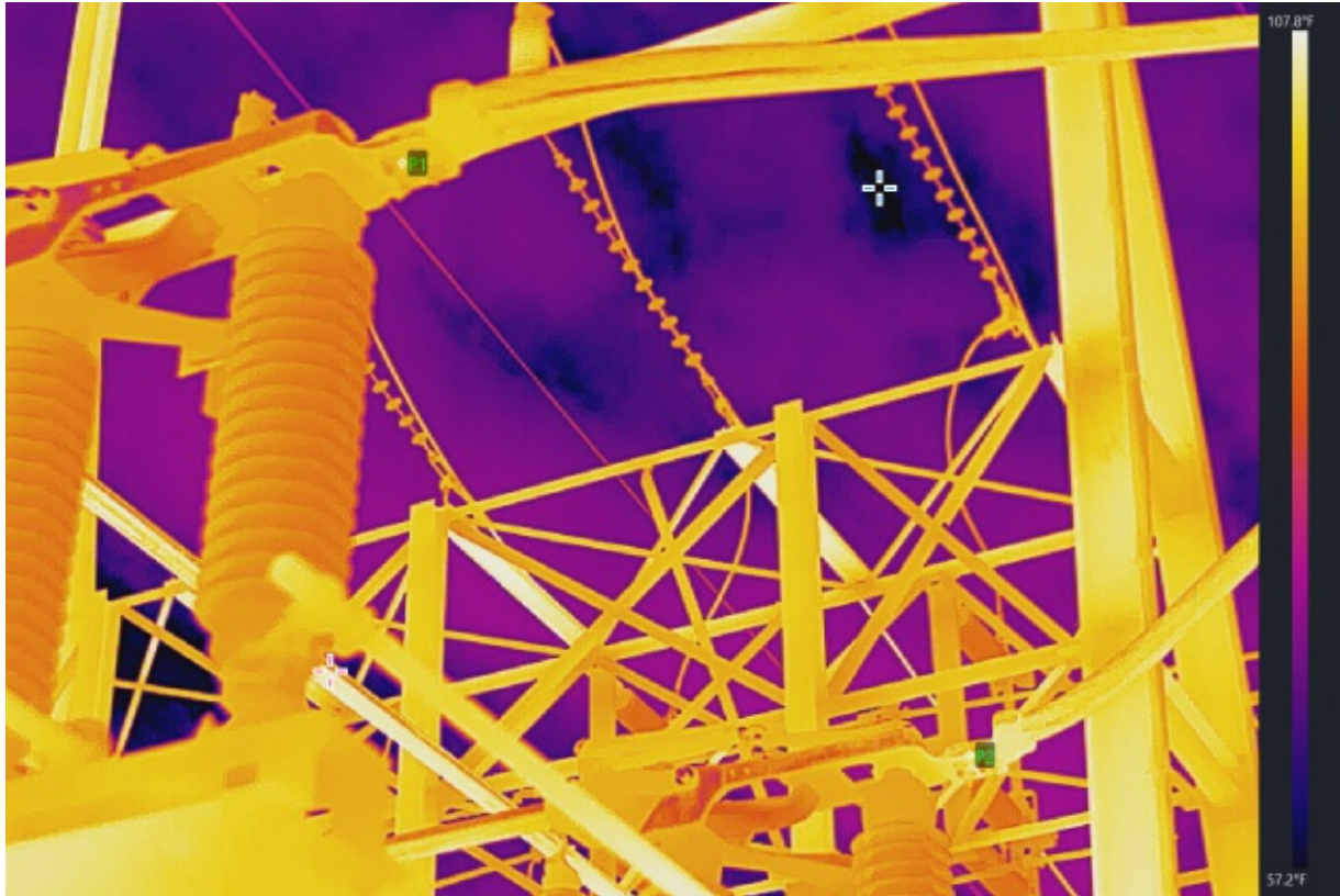
T2 - MAIN AIR SWITCH
