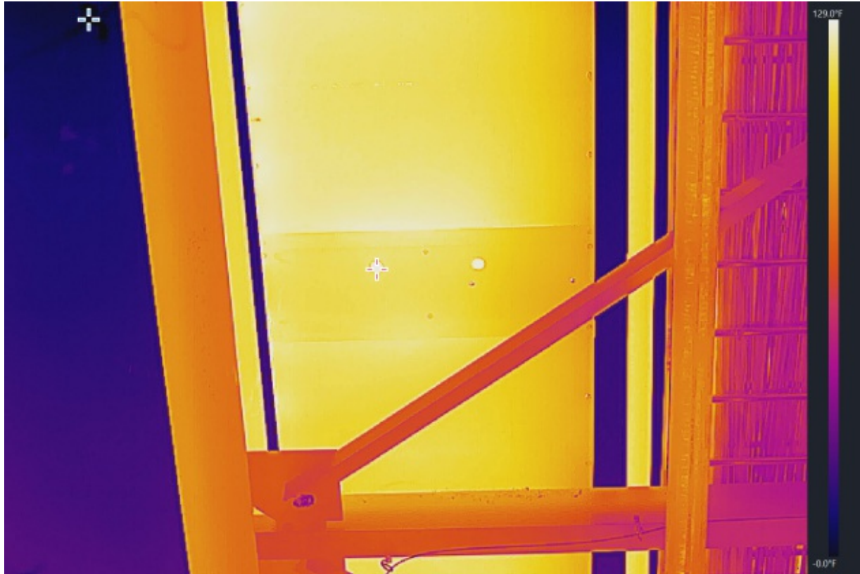
BUS DUCT HEATERS
