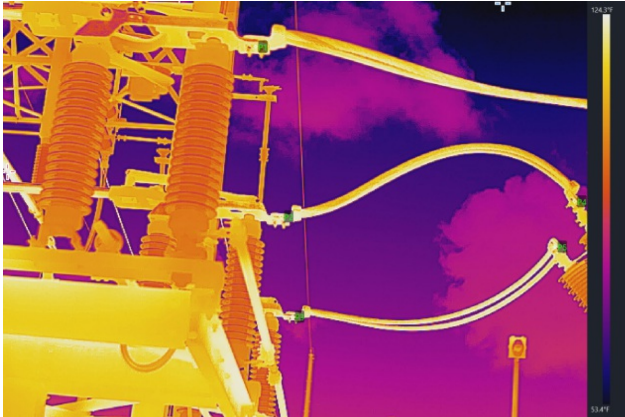
T2 - MAIN AIR SWITCH
