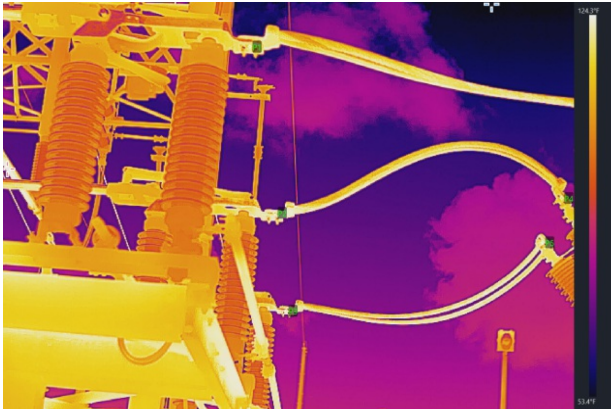
T2 - MAIN AIR SWITCH
