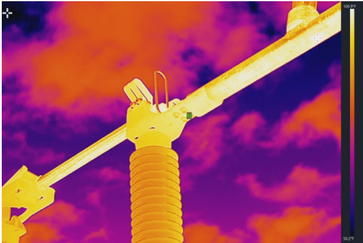
T2 - MAIN AIR SWITCH
