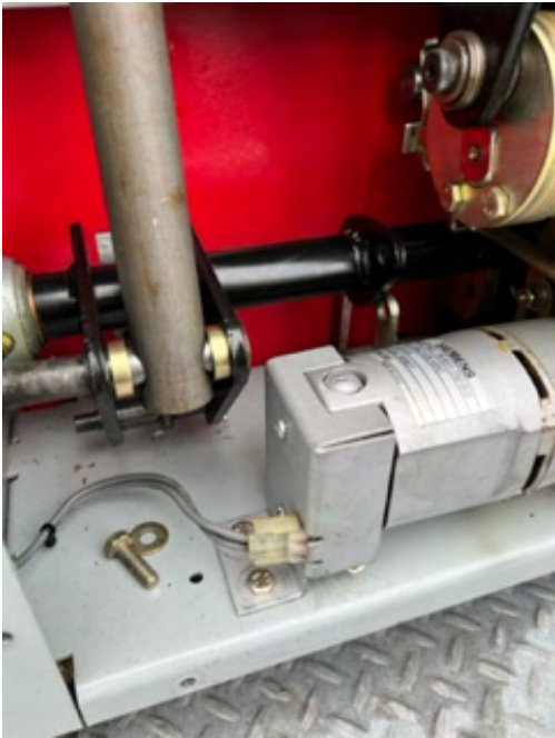
Bolt was not in place for breaker to be racked out and closing latch to be in the up position
