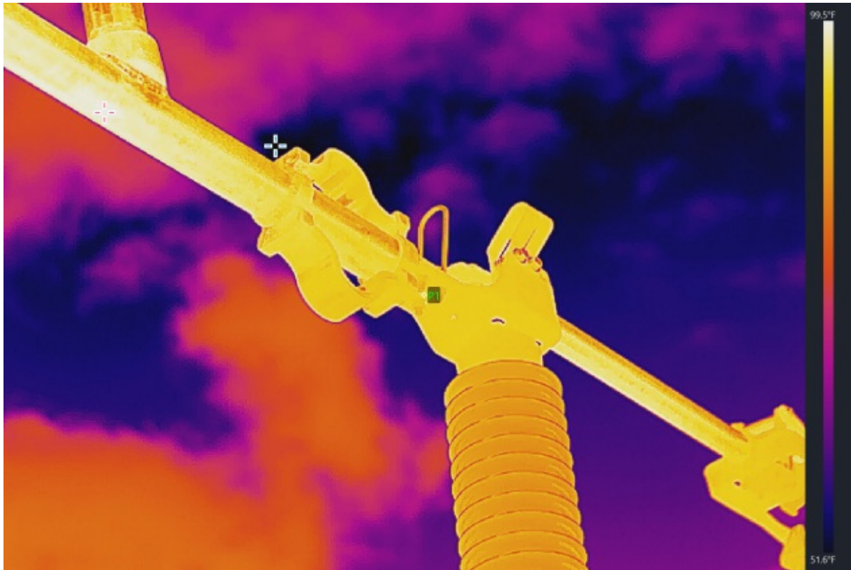
T1 - MAIN AIR SWITCH
