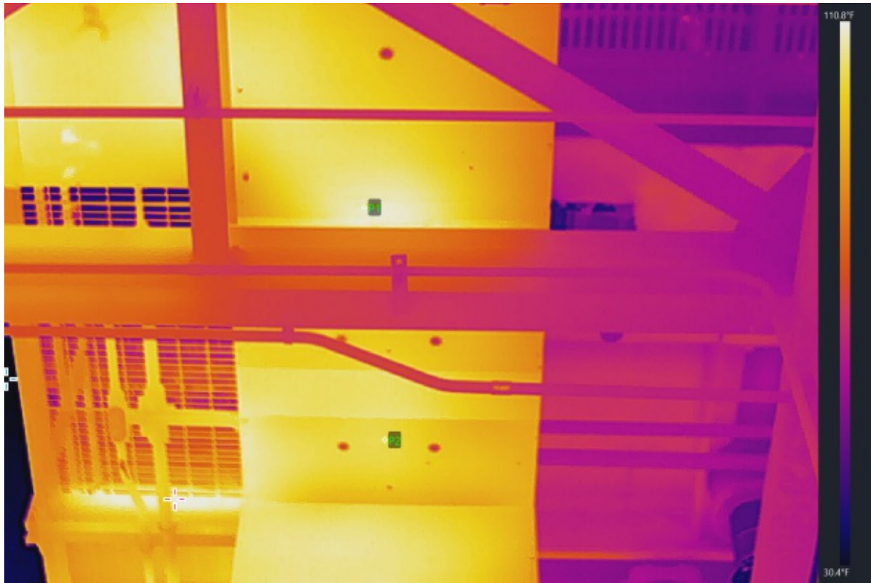
BUS DUCT HEATERS
