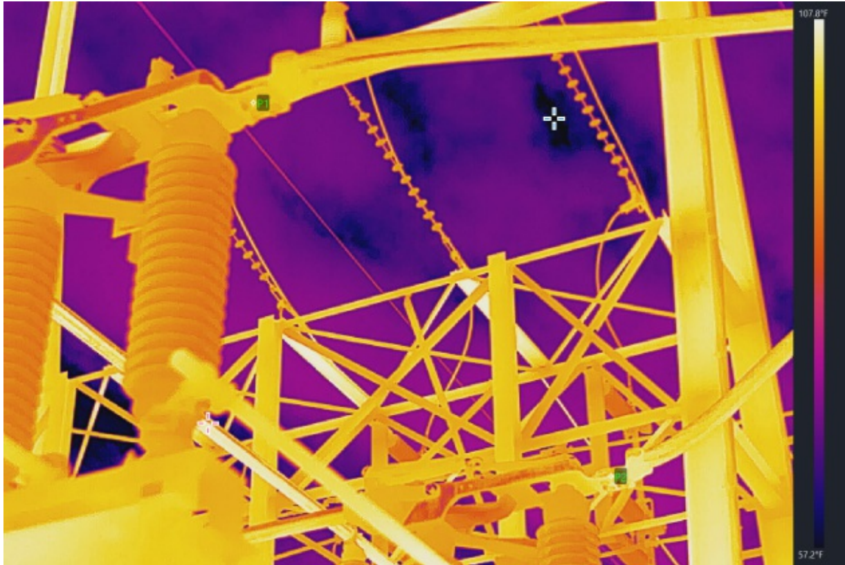
T2 - MAIN AIR SWITCH
