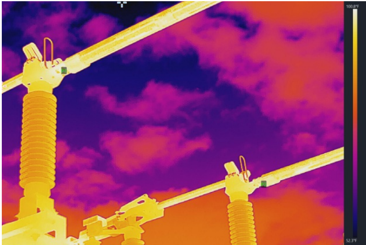
T2 - MAIN AIR SWITCH
