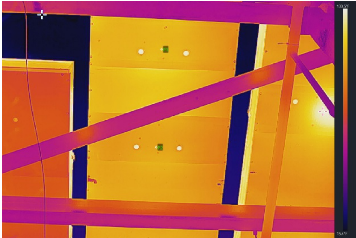
BUS DUCT HEATERS
