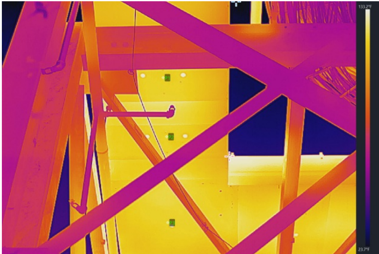
BUS DUCT HEATERS
