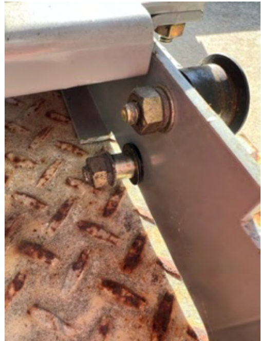
Wheels should be attached here, but broke off
