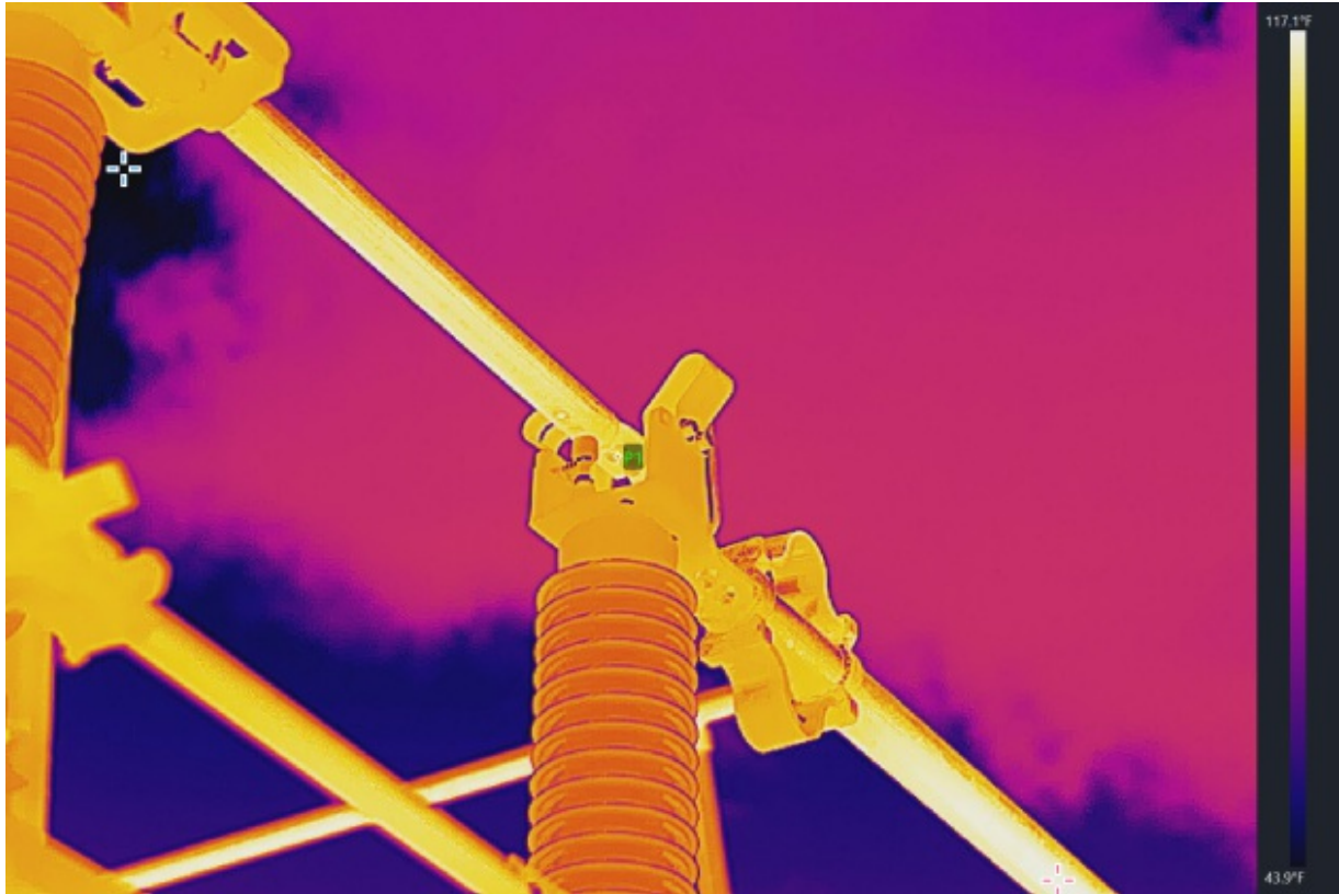
T1 - MAIN AIR SWITCH
