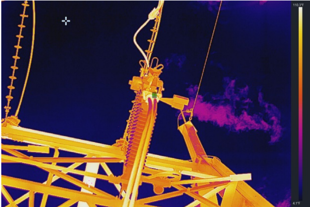
SWITCHYARD MAIN SWITCH
