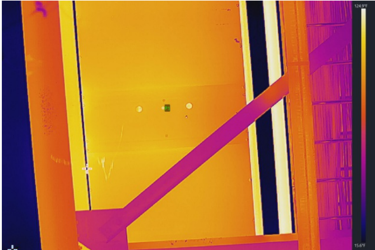
BUS DUCT HEATERS
