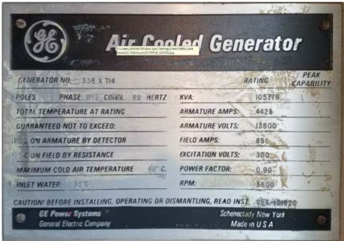
Figure 2: CIPP CT2 Generator Nameplate
