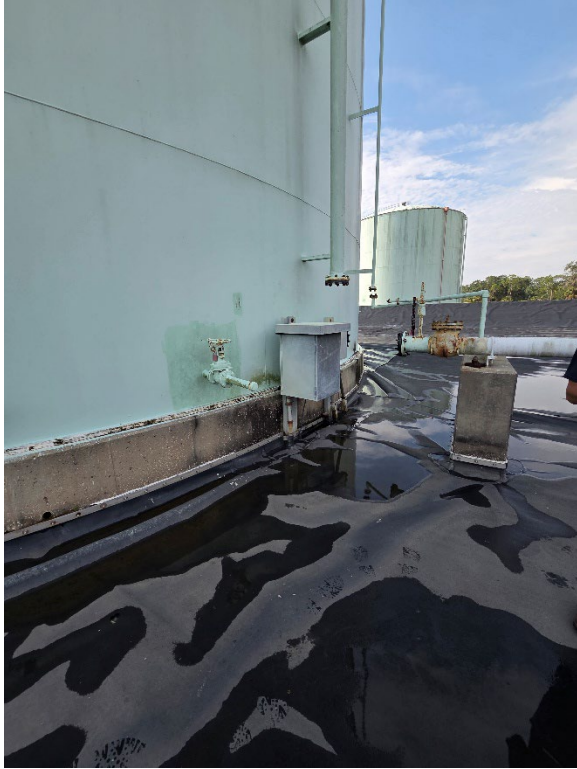
Figure 6: Cathodic Protection General
