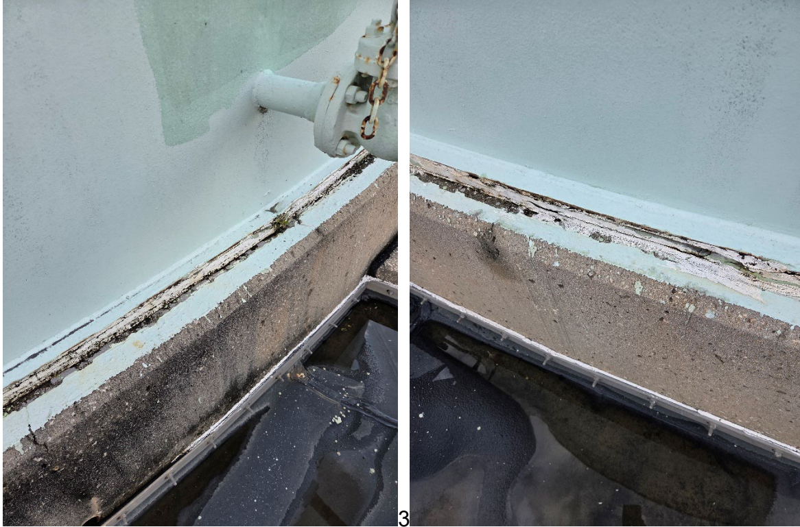
Figure 5: Typical Chime Condition
