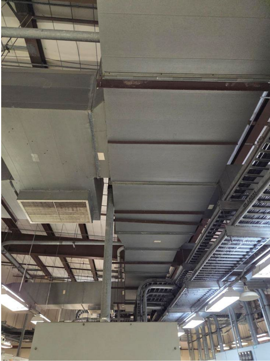
Figure 8: Supply Trunk in MCC Room
