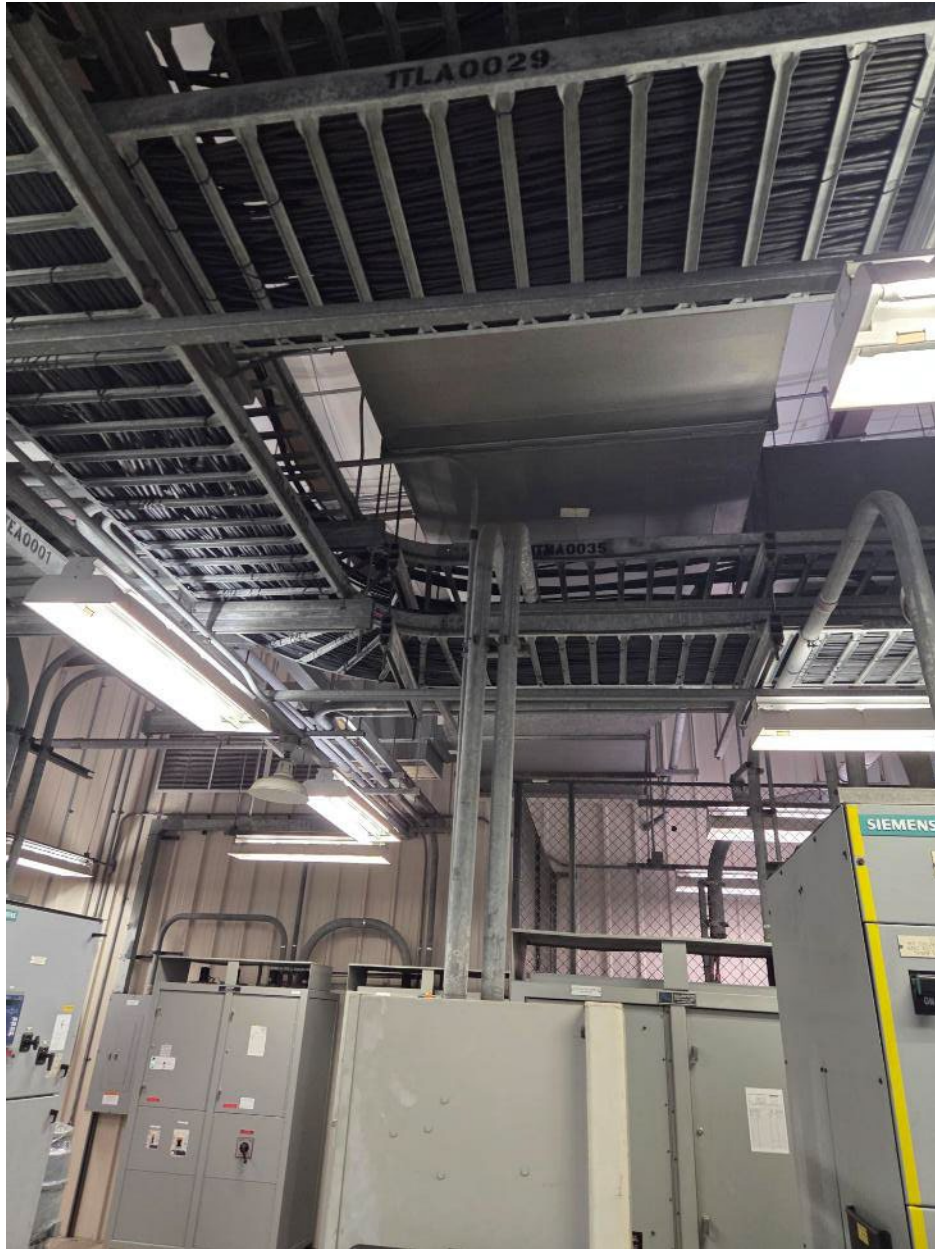
Figure 7: Supply Trunk in MCC Room
