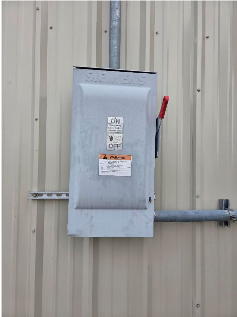
Figure 4: Existing 480V, 3-Phase Service Disconnect
