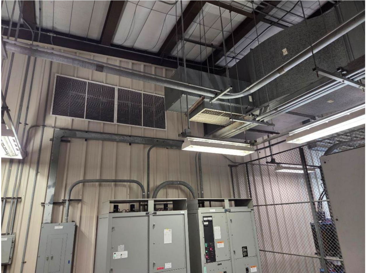
Figure 6: Return and Supply Ductwork Inside MCC Room
